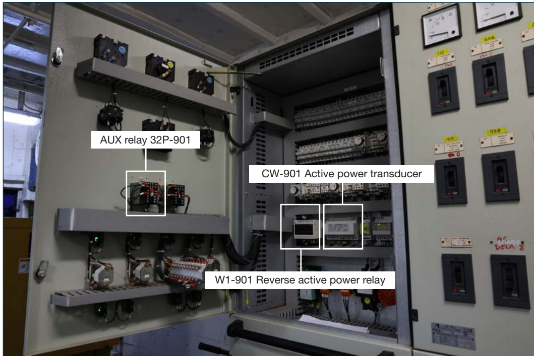
Figure 51: Reverse power protection units in emergency switchboard cabinet. Source: DMAIB
