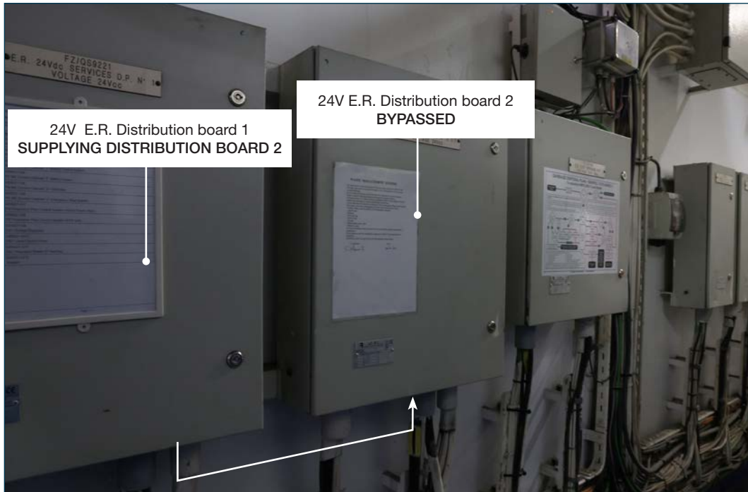
Figure 53: Distribution board for 24 V services in engine room bypassed. Source: DMAIB
