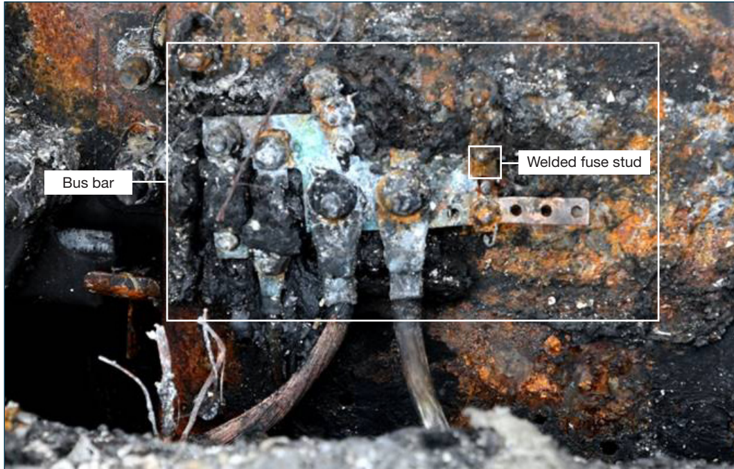
Figure 23: Remains of fuse box bus-bar. Source: DMAIB
