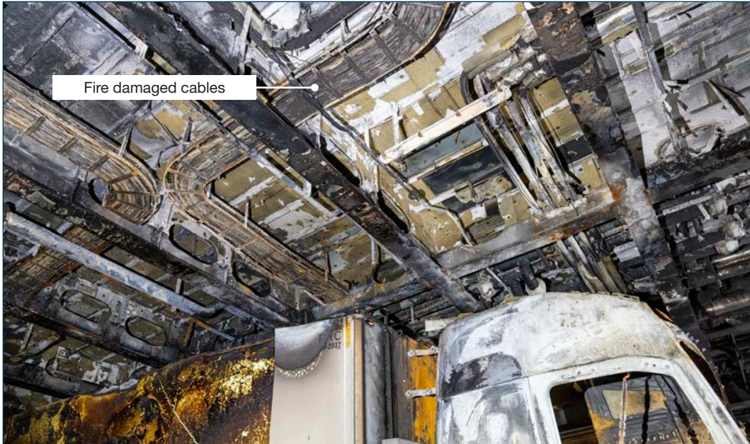
Figure 36: Fire damages to the deck head above the burning truck. Source: DMAIB
