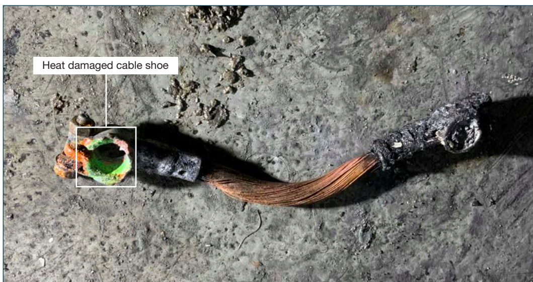
Figure 29: Heat damaged cable shoe on battery wire connection.
