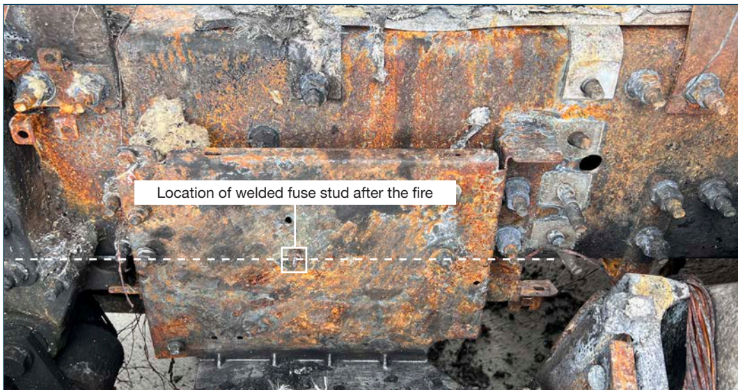
Figure 31: Heat damaged cable shoe on battery wire connection. Source: DMAIB
