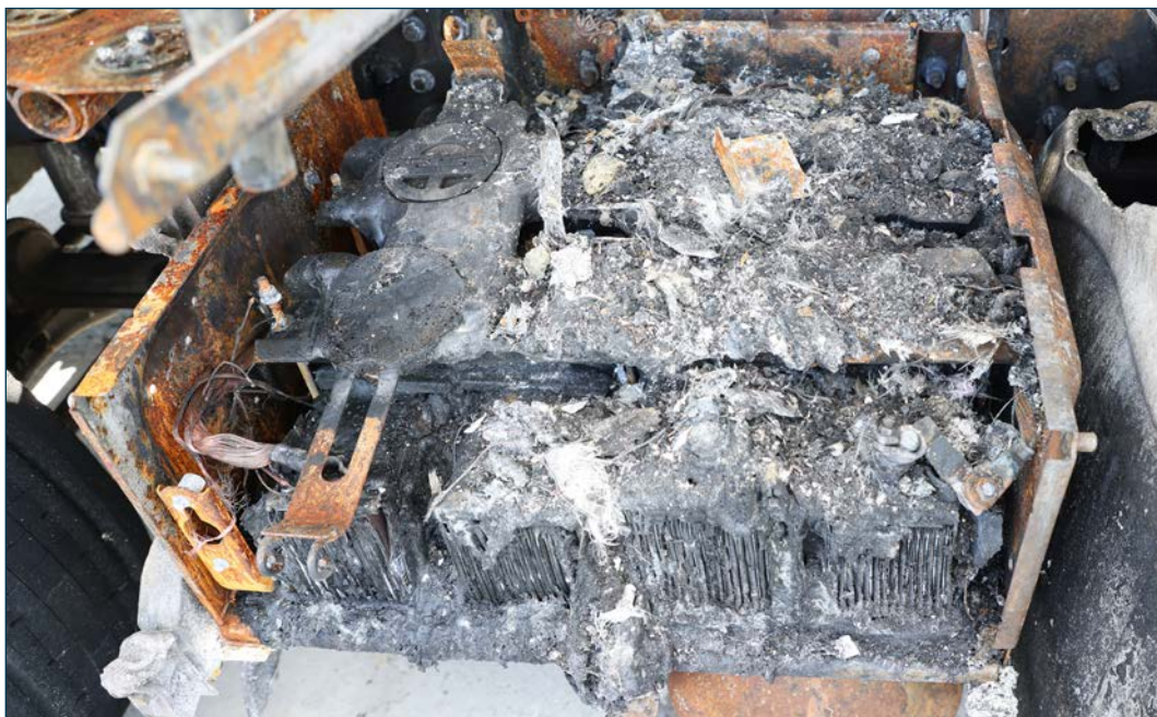
Figure 27: Damaged starter battery. Source: DMAIB
