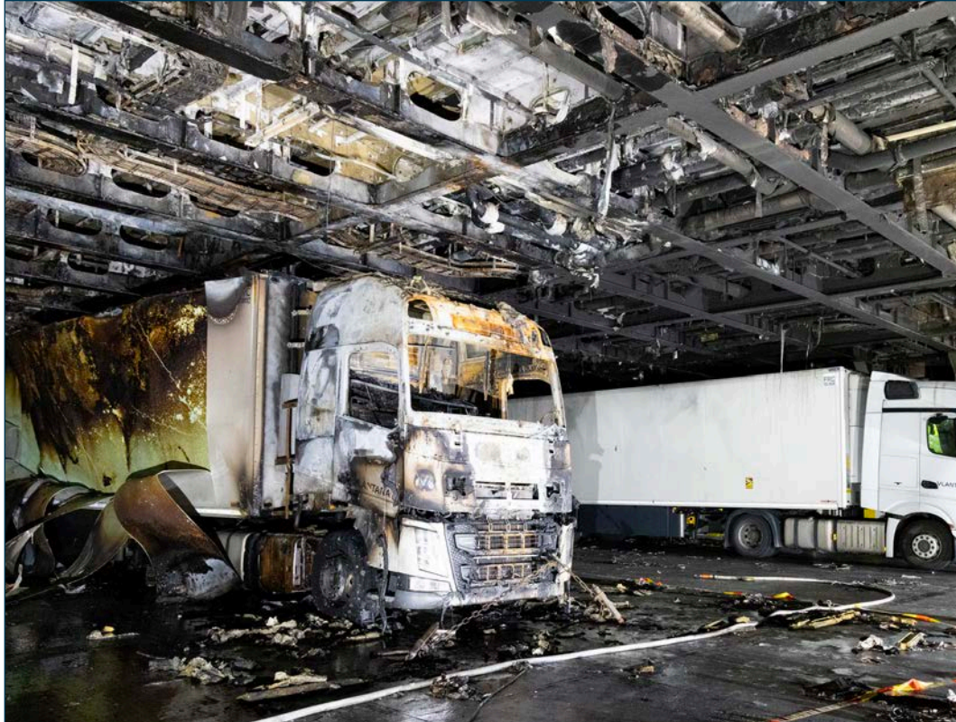
Figure 14: Deckhead above truck burnt clean from paint and soot. Source: DMAIB
