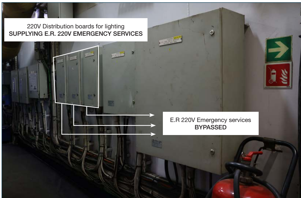
Figure 54: Distribution board for 220V emergency services in engine room bypassed. Source: DMAIB
