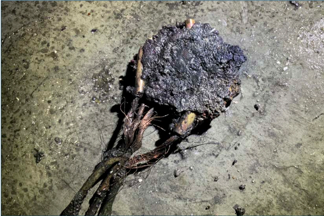
Figure 21: Melted power cable inlet. Source: DMAIB
