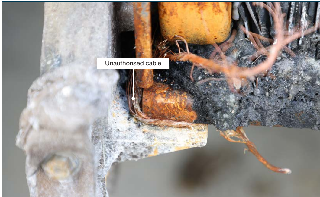
Figure 28: Unauthorised power installation.
