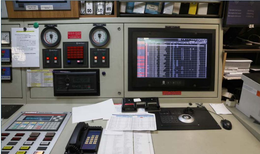
Figure 44: Monitor for alarm monitoring system. Source: DMAIB
