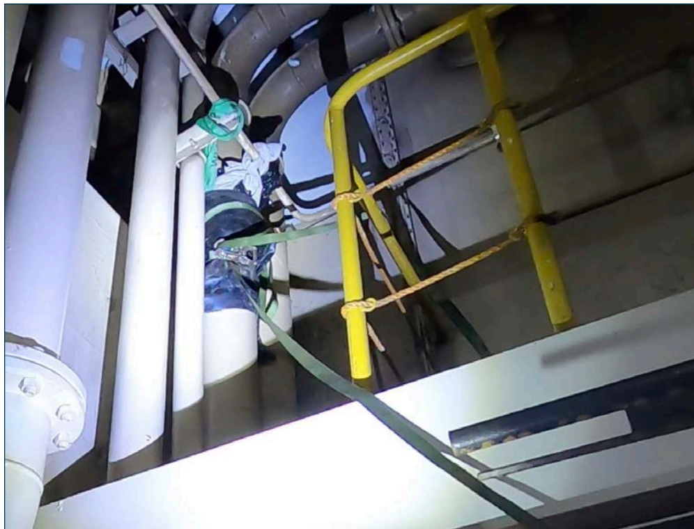
Figure 9: Sealed off drencher pipe leakage. Source: DMAIB
